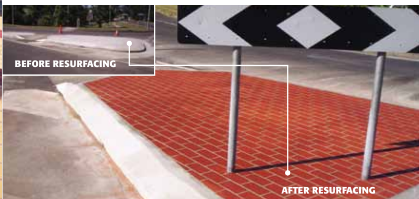
Stylepave Resurfacing is a low maintenance, cost effective way to spruce up traffic islands and roadways.
